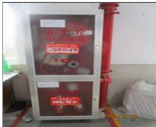
Photo of fire safety equipment Fire equipment.JPG
