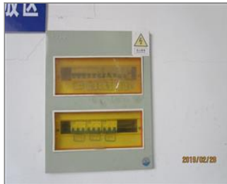
Photo of the inside of the main production hall Control panel with safety warning.JPG
