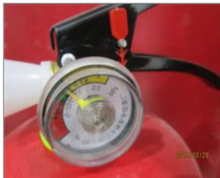
Photo of fire safety equipment Fire extinguisher in proper in pressure.JPG
