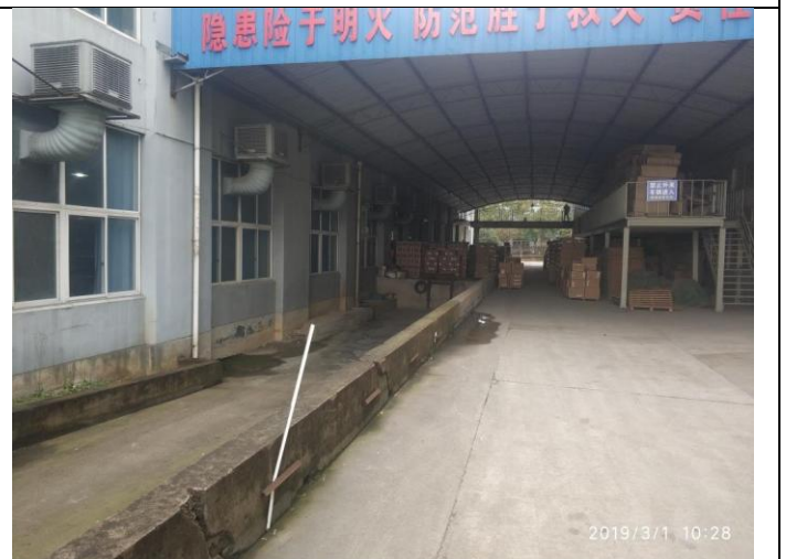
NC Findings description: Facility did not have proper fencings to enclose cargo handling and storage areas to prevent unauthorized access.
